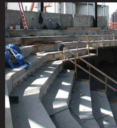
DIFFUSER OPENINGS BENEATH EACH SEAT ©MCGOUGH
